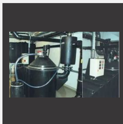
Grease separator for self-disposal
